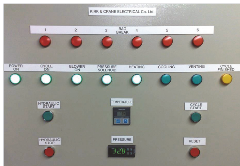
Figure 7-3: Control panel – clear layout and markings.
