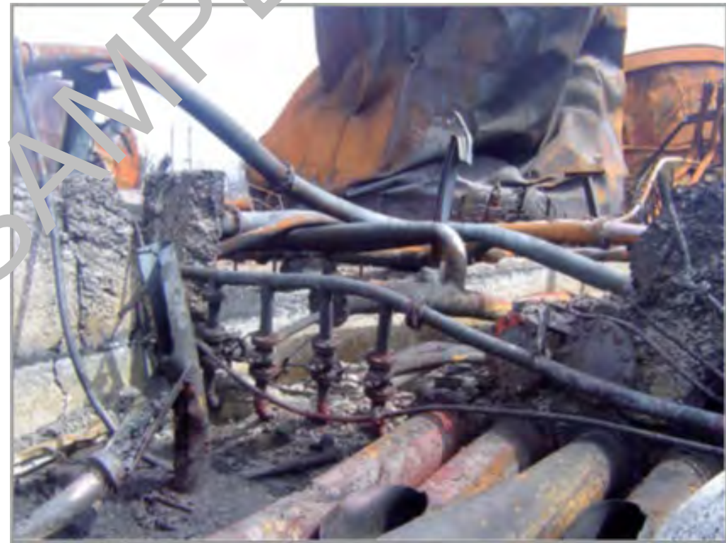
Catastrophic bund wall failure at pipe penetrations
