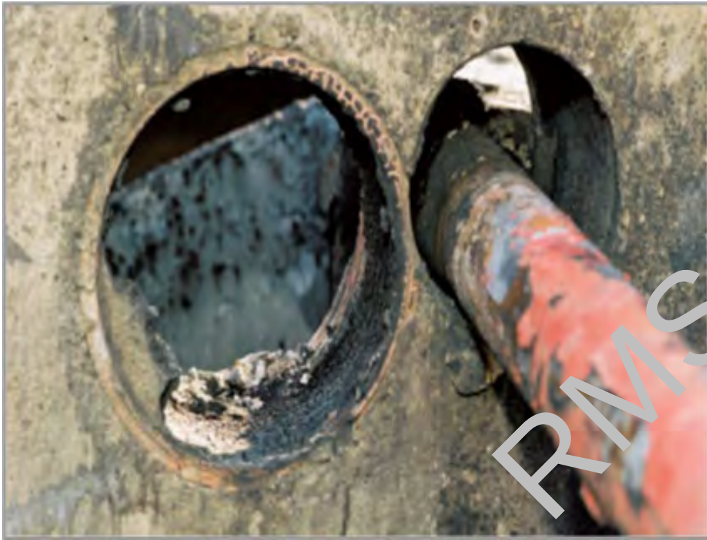
Loss of sealant between penetrating pipe and bund wall.
